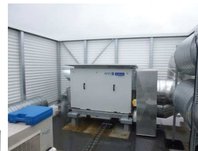
VENTILATION DOUBLE FLUX
